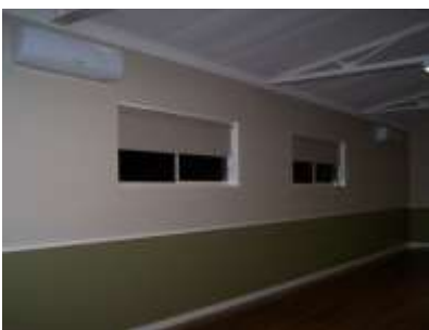
Split systems (installed in Hall & Supper Room)
