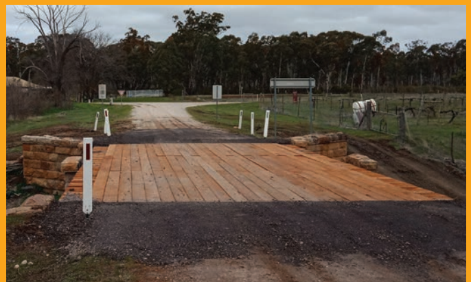
Rehabilitation works to Kingower Brenanah bridge at Kingower were completed at the end of August, including a new timber deck.
